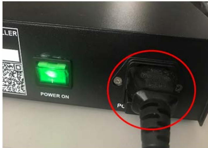
Figure 4 – FDC Power cable
