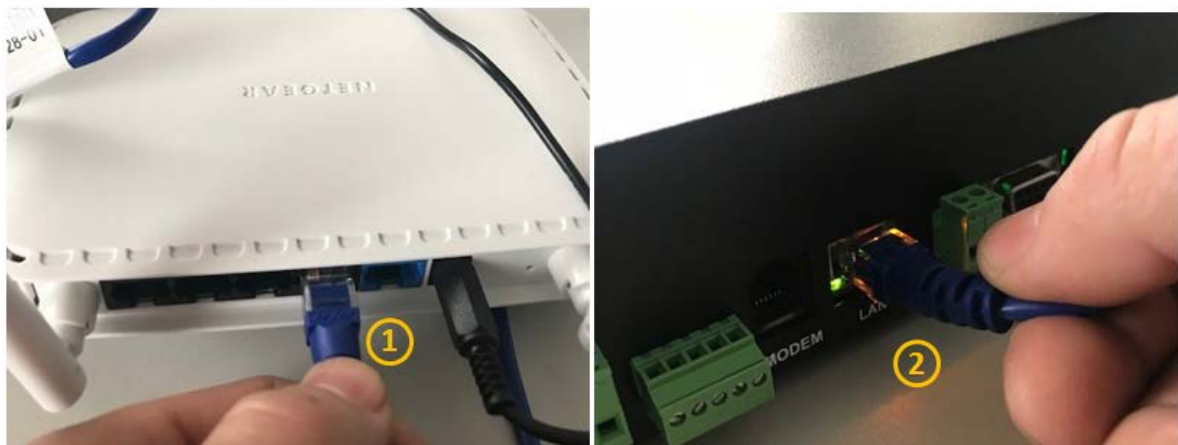
Figure 5 – Router and FDC patch cable connection
